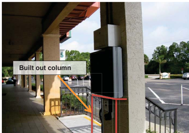
Sign is a protruding object
