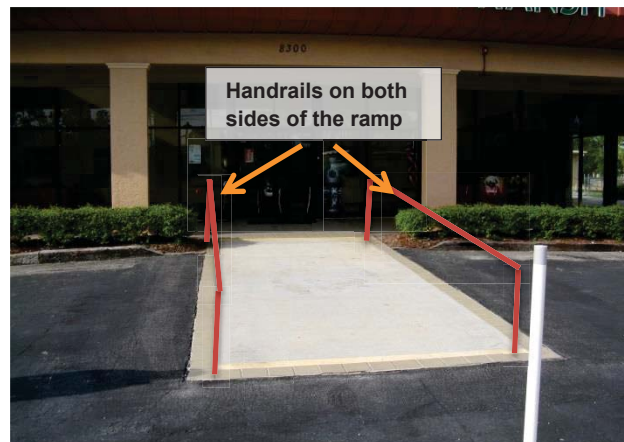
Incompliant entrance ramp slope
