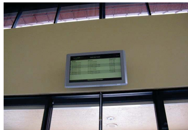
Incompliant character heights
